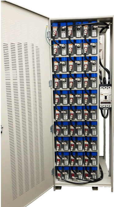
Three string XLM-62 supercapacitor module cabinet shown above
