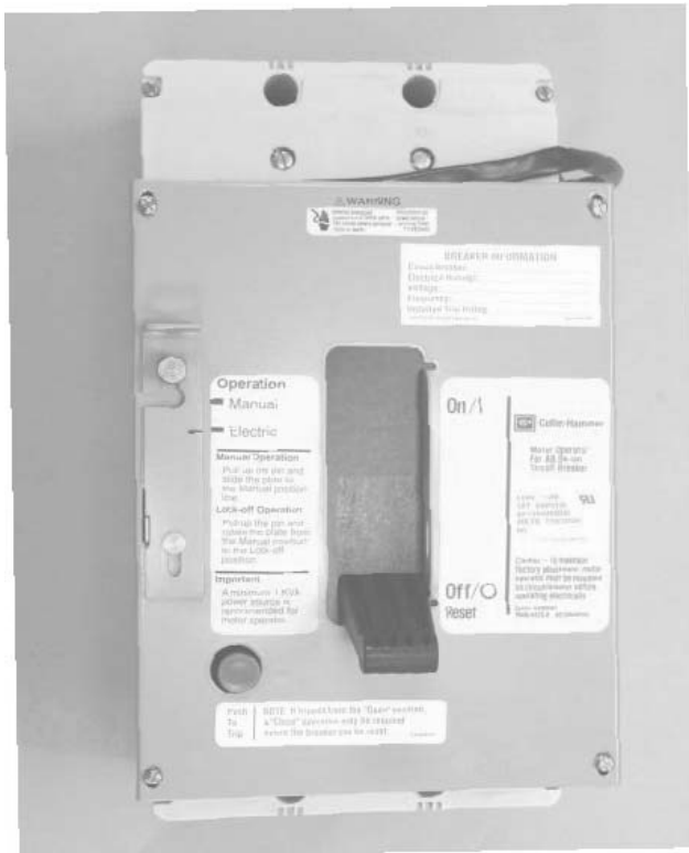
Fig. 3-2. Motor Operator in Electrical Position
