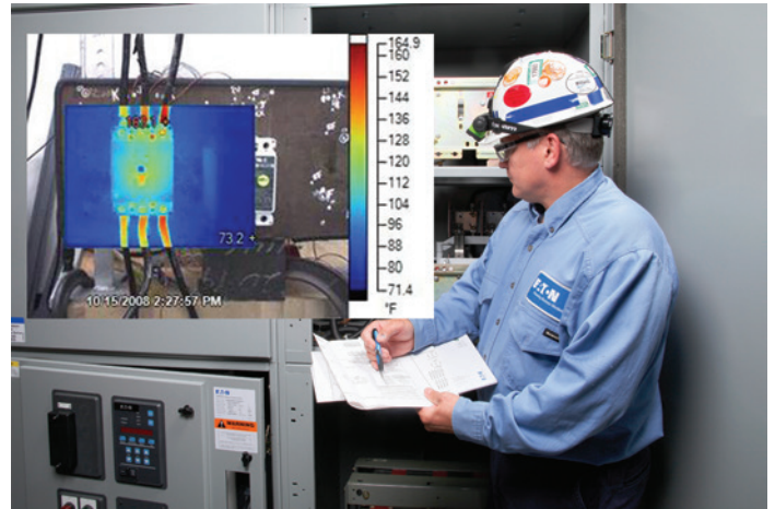
Figure 4. IR cameras can be used to provide insight to see breaker health.
