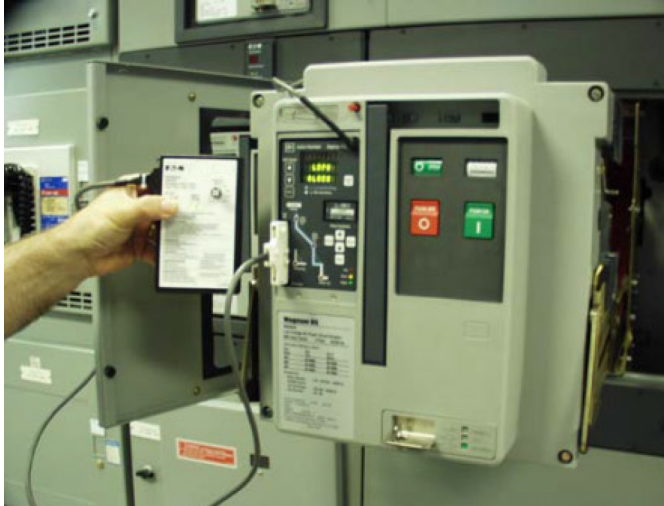
Figure 5. Testing Digitrip 1150 with Magnum Breaker in Disconnected Cell Position.
