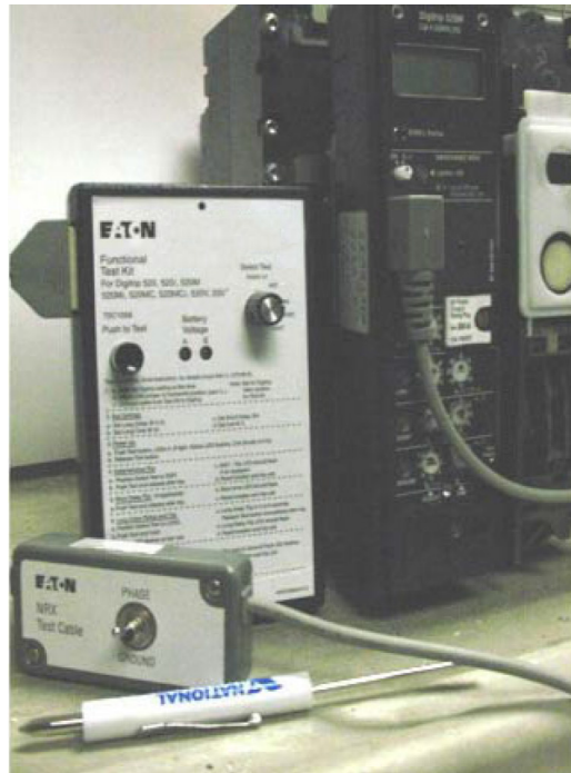
Figure 7. Testing a Series NRX Circuit Breaker.
