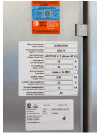
The labels indicate that the switch cabinet was approved by ESA inspectors (Electrical Safety Authority).
