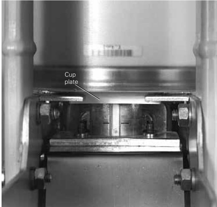
Figure 28. Vacuum interrupter showing contact erosion indicator with breaker open (shown here for clarity purposes only).
