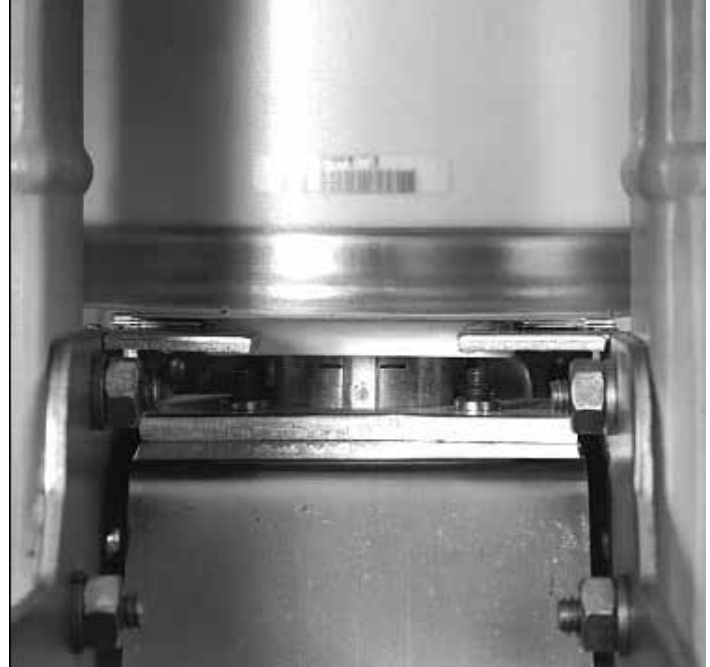
Figure 29. Vacuum interrupter showing contact erosion indicator with breaker closed (indicators are checked only when the breaker is closed).
