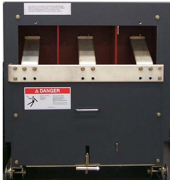
Figure 1: Device shown with upper terminals grounded Torque .375-16 (Grade 5) Hardware to 20ft./lbs.
