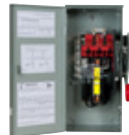
DC safety switches
