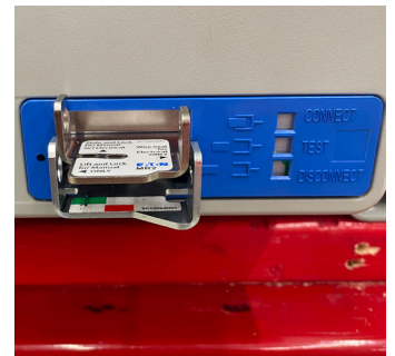
Figure 14. Door lifted and held up.
