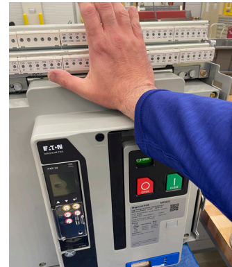
Figure 3. Tertiary connection in disconnect.
