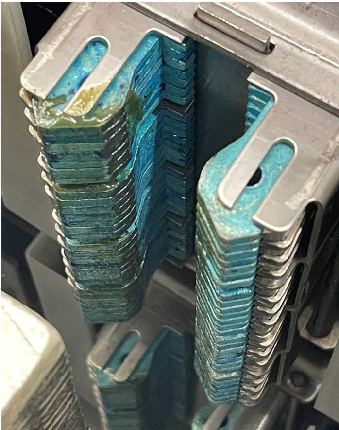
Figure 26. Magnalube applied to the primary disconnects.
