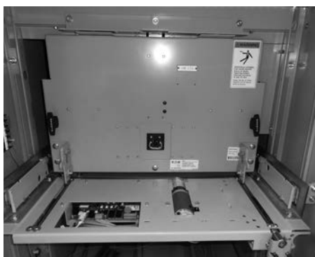
Type VC-W Standard Switchgear Auxiliary Drawer with Type MR2 Integral Racking
