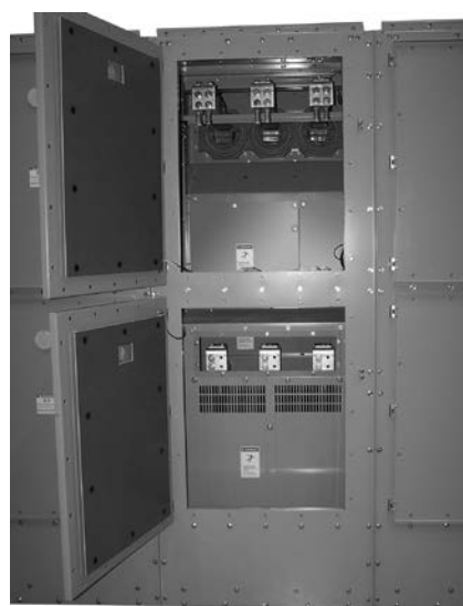
Rear View— Breaker Over Breaker Cable Termination
