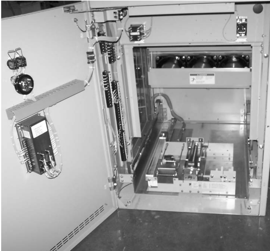
Roll-on-the-Floor Switchgear Compartment
