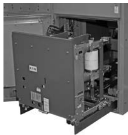
Breaker Shown Fully Withdrawn on Extension Rails
