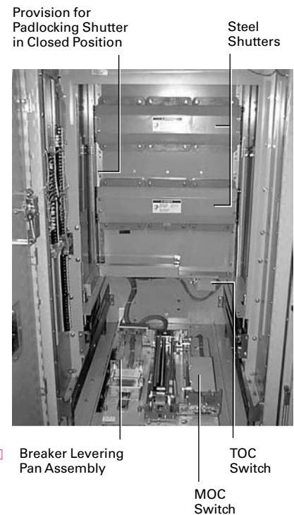
38 kV Switchgear—Circuit Breaker Compartment
