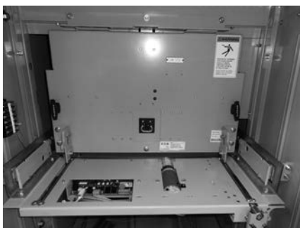
Type VC-W Standard Switchgear Auxiliary Drawer with Type MR2 Integral Racking
