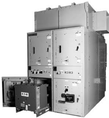
Arc-Resistant Switchgear with Plenum Installed
