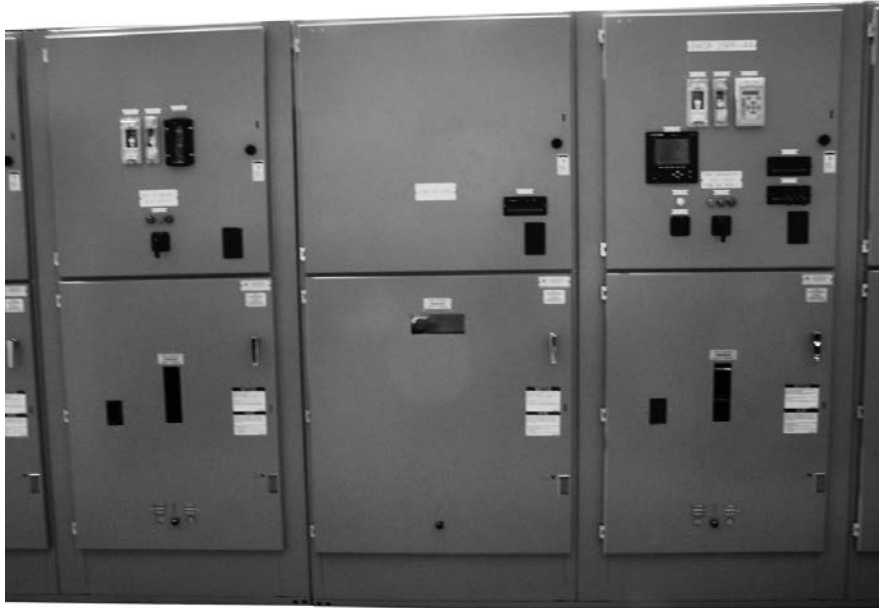
Front View—27 kV VCP-W Arc-Resistant Switchgear (Plenum Above the Switchgear is Not Shown)
