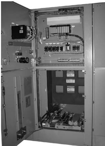
Typical 27 kV Cell—Controls in Top, Breaker in the Bottom
