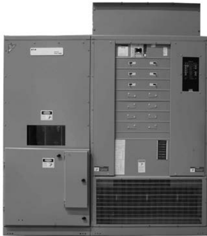
Unitized Power Center
