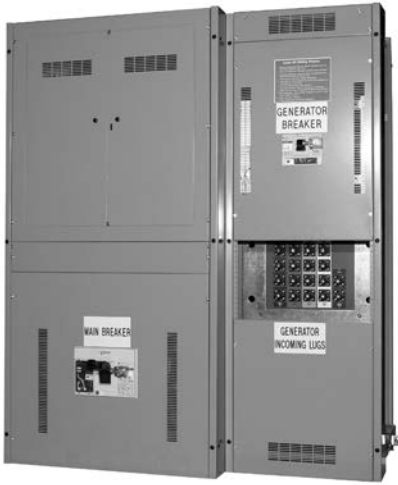
Generator Quick Connect Switchboard Section
