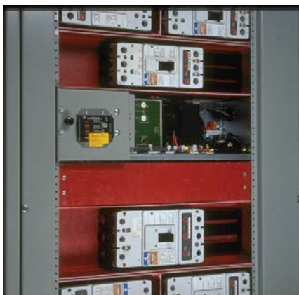
Ground fault test panels can be mounted in compartments with the circuit breakers for convenience and space savings.
