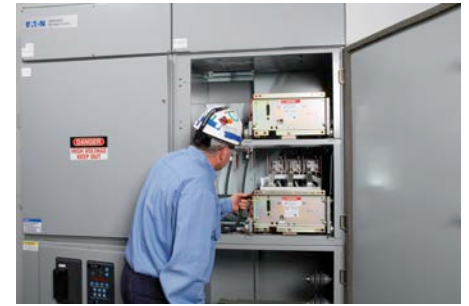
Arcflash Reduction Maintenance System (ARMS)
