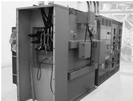
VFI with Secondary Unit Substation
