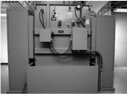
VFI Primary with Secondary Cable Connections and Containment Pan
