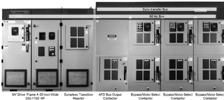
Synchronous Transfer Control System
