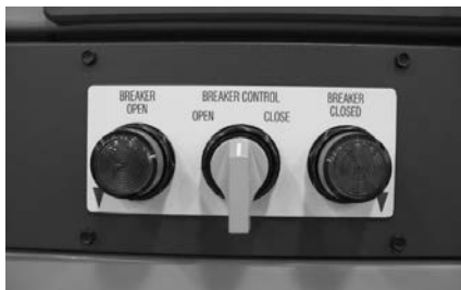
Devices Mounted on Secondary Terminal Compartment Door
