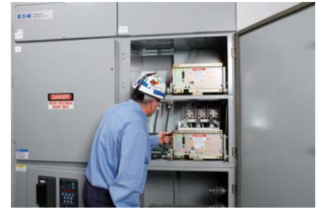
Arcflash Reduction Maintenance System (ARMS)
