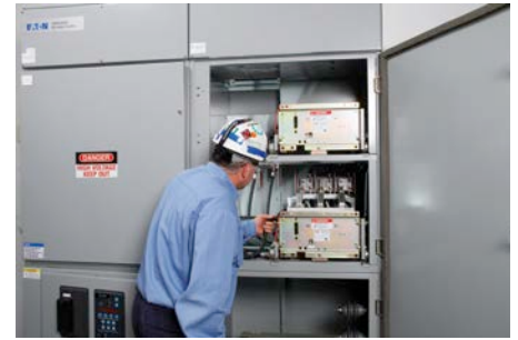
Arcflash Reduction Maintenance System (ARMS)
