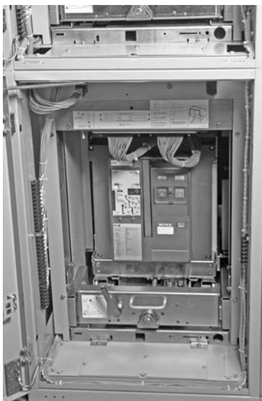
Circuit Breaker Compartment— Breaker in Connected Position
