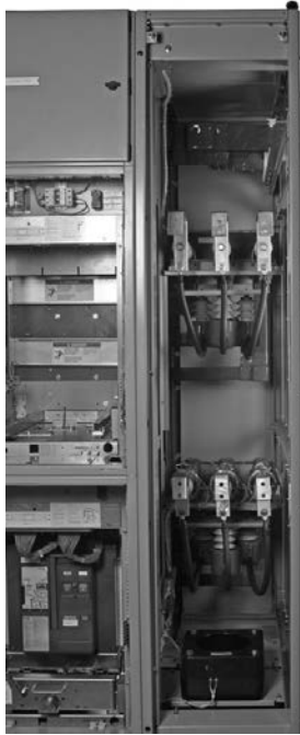
MEF Cable Pull Section Adjacent to 2-High Breaker Cell
