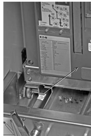
Circuit Breaker in Connected Position Indicator
