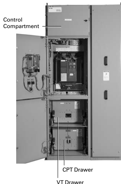
MEF Switchgear—Indoor Unit
