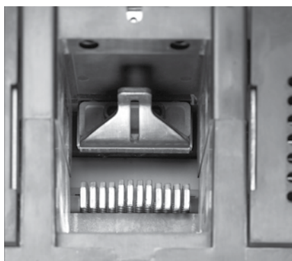
Magnum DS Breaker Contacts (Arc Chutes Removed)
