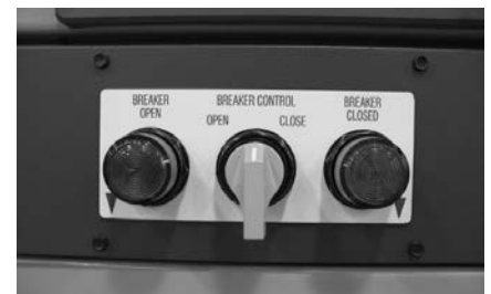
Devices Mounted on Secondary Terminal Compartment Door
