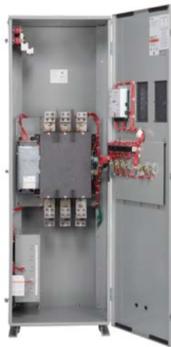
Automatic Transfer Switch (ATS)
