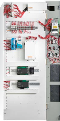
Safe, easy and spacious access to wiring and components.
