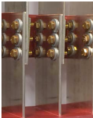
Bypass isolation ATS—close-up of configurable bus
