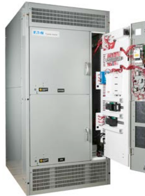
Control compartment door and adjoining electrical panel slide forward.
