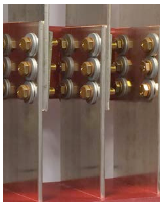
Bypass isolation ATS—close-up of configurable bus
