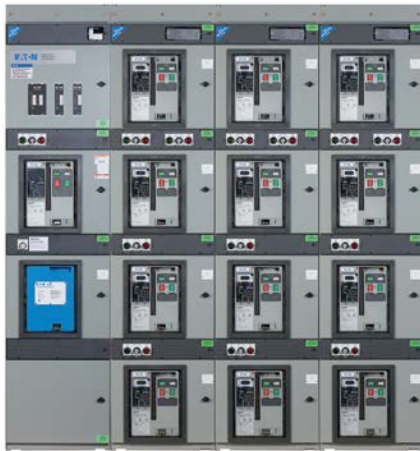
Arc Quenching Switchgear
