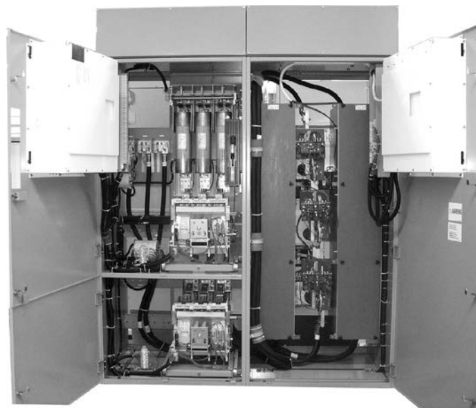
720 A MV4S with Doors Open
