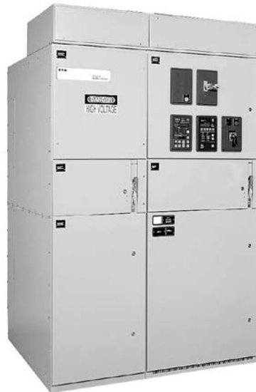
Main Breaker Ampgard
