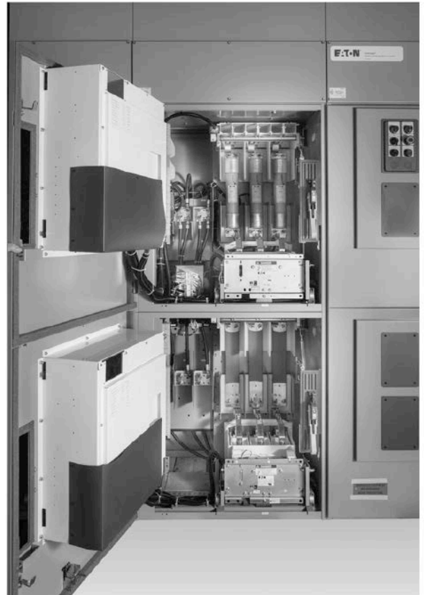
400 A Stacked with VFD Bus
