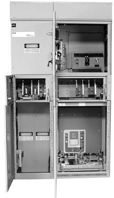
Main Breaker Ampgard—Doors Open
