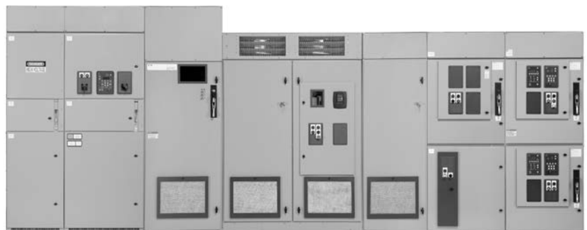
Ampgard Main Breaker
