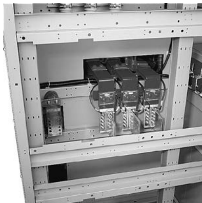
Side Panel Removed to Show Incoming Cable Connections
