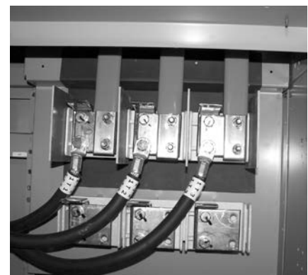
Load Cables—Moved for Full Voltage Start
