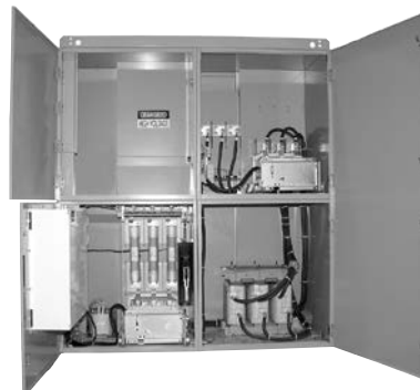
Reactor Starter Shown in Non-Arc Enclosure
