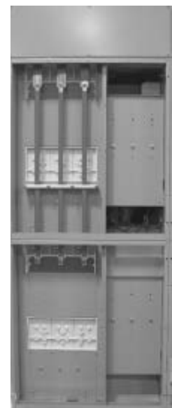
Vertical Bus, Rear View (2-High 400 A) Shown in Non-Arc Enclosure
