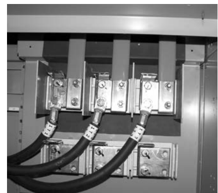
Load Cables—Moved for Full Voltage Start
