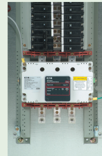
In this installation, the SPD Series is mounted directly to the panelboard's bus bars. This type of installation will provide the best possible surge protection by minimizing the connected lead length.
