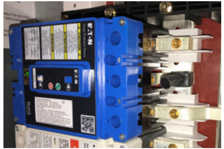
Figure 5. SPD installed - terminal side.
