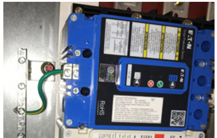
Figure 6. SPD installed - surge ground terminal.
