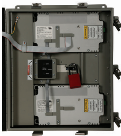
SPM Series devices include industry exclusive barriers and lockout provisions to mitigate arc flash exposure.
