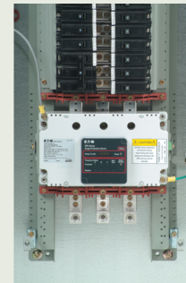
In this installation, the SPD Series is mounted directly to the panelboard's bus bars. This type of installation will provide the best possible surge protection by minimizing the connected lead length.
