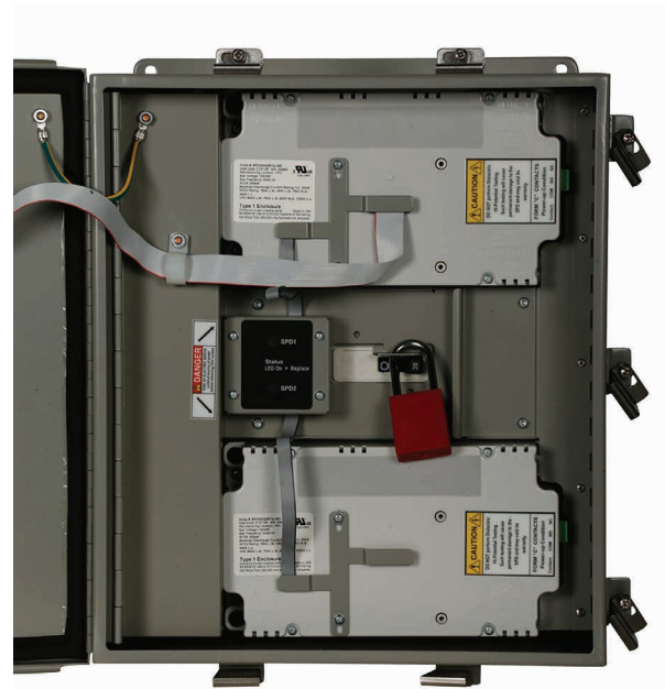
SPD MAX with safety barriers and optional circuit breaker locked out
