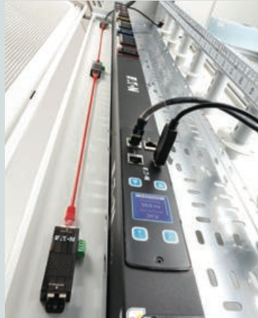
Three daisy-chained environmental monitoring probes with a rack PDU
