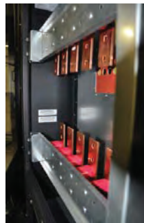
Figure 14. Reserve and Load Power Cables
