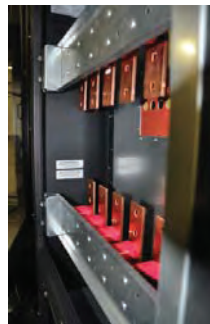
Load (Busway) Bus Bars
