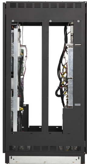
Rack RPP, side view
