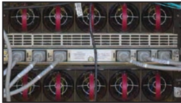
Typical server with multiple power inputs powered by two rack PDUs
