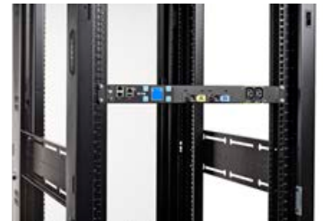
Here is an example of a horizontally-mounted 1U PDU.
