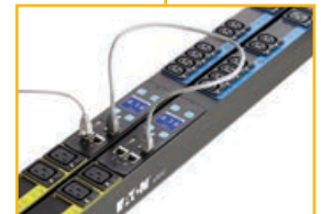
A and B power PDU sharing a network connection via daisy chain
