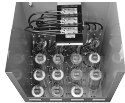
UNIPAK Capacitor Bank Interior
