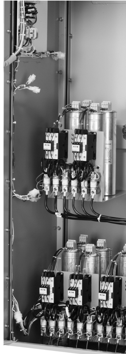
Factory Pre-Wired for Future Expansion
