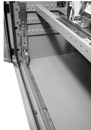
Continuous Ground Bus with Pad in Each Section
