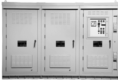
Safety and Aesthetics are Just Two Compelling Reasons to Use Metal-Enclosed PFC Systems
