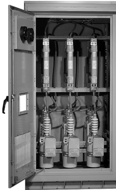
15 kV Switched Capacitor Stage Enclosure
