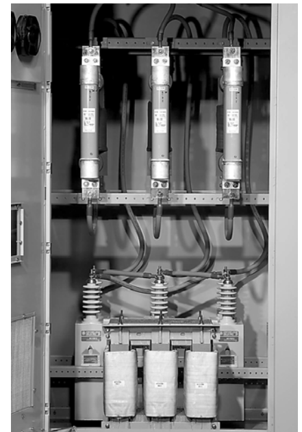
Detuned Filter Capacitor Stage Enclosure
