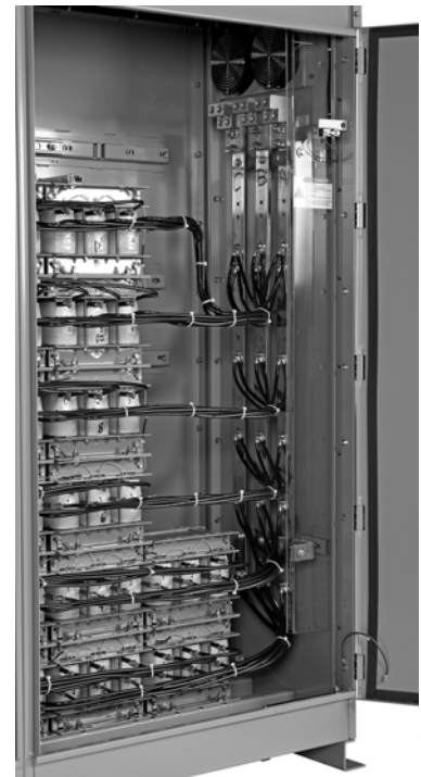
AUTOVAR Filter—Reactor Cabinet
