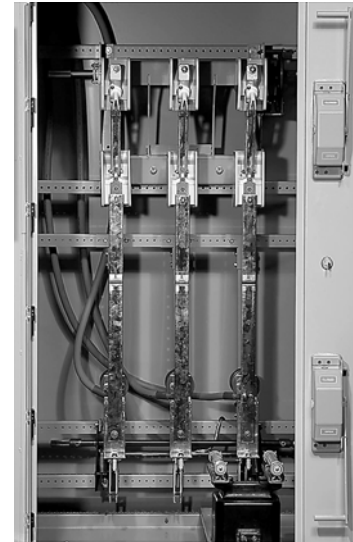
Incoming Main Switch and Fuses
