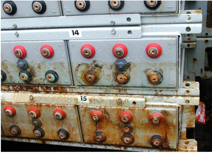
Electrical equipment destroyed during Hurricane Sandy
