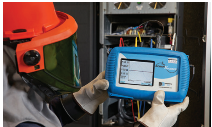
A power quality meter records voltages, currents, and harmonic content at the output of a UPS to identify irregularities in the waveform caused by electrical issues.
