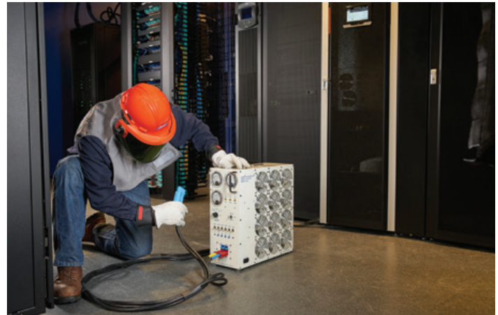
A load bank test simulates maximum load conditions so you can check performance and runtime at increasing load levels.
