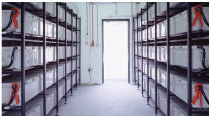
Eaton Cellwatch battery monitoring system monitors key performance indicators for each individual battery to provide adequate time to detect and replace a bad battery, mitigating the risk of downtime
