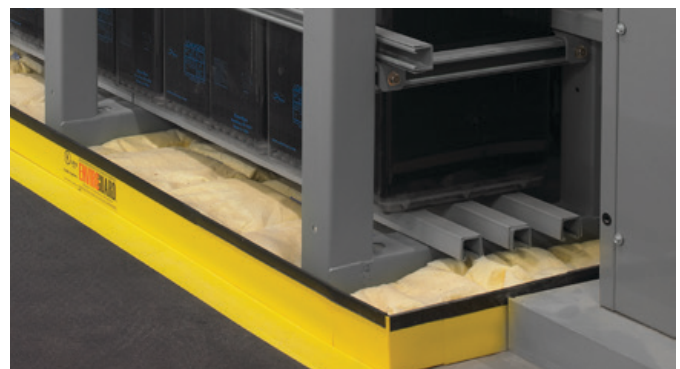
Battery spill trays are designed to contain and absorb leaking batteries
