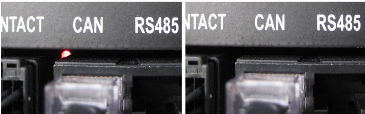
Figure 4-1. System BMS LED
