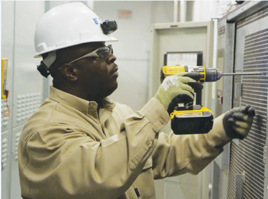
An Eaton service technician performs maintenance on one of Windstream's 10 Eaton UPSs.
