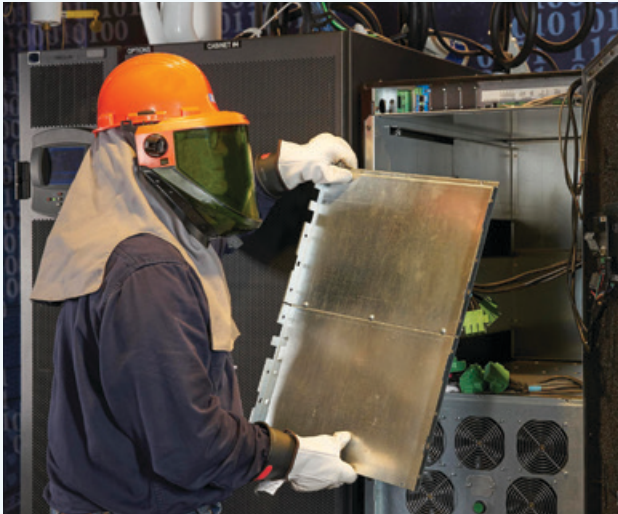
Proper preventive maintenance reduces the risk of UPS failure through thorough inspection, cleaning, testing and calibrating various electronic and mechanical components.
