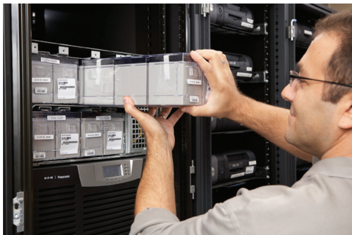
Figure 8. Hot swappable battery modules allow service work to be performed while load equipment remains protected.
