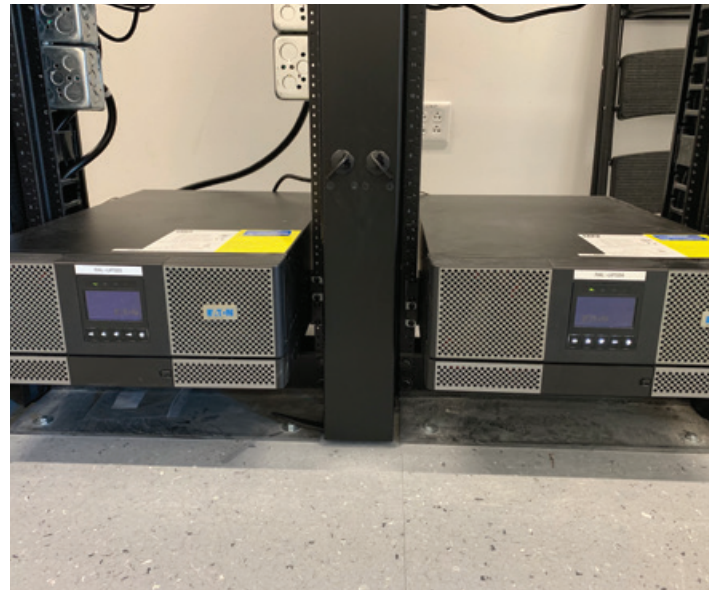
Two Eaton 9PX UPSs protecting Stewart's servers and other critical devices.
