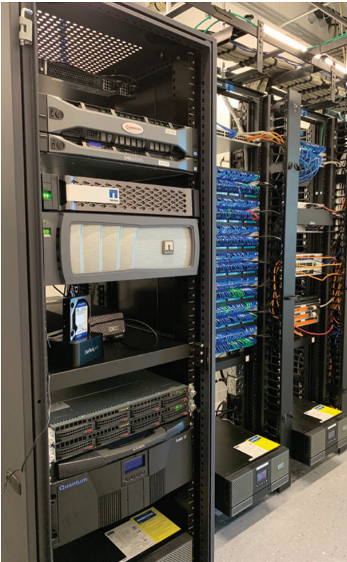
The server room at Stewart's new office.
