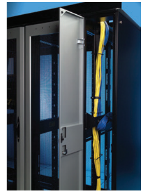
Side cable management channel
