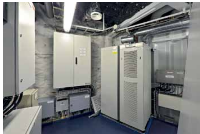
Eaton 9355 Marine UPS on board Allure of the Seas
