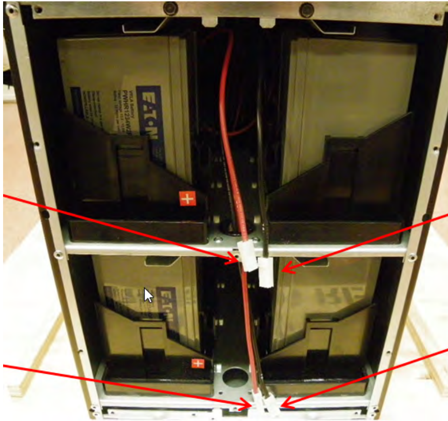
Figure 7. Disconnected Cabinet Harnesses
