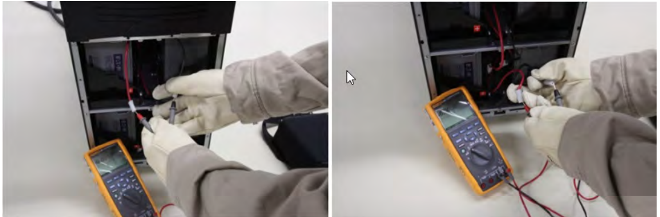
Figure 8. Verify Zero Voltage
